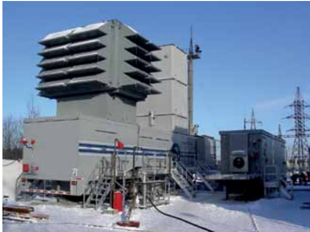
Pratt & Whitney Power Systems FT8 MOBILEPAC® Daryino, Moscow Region
